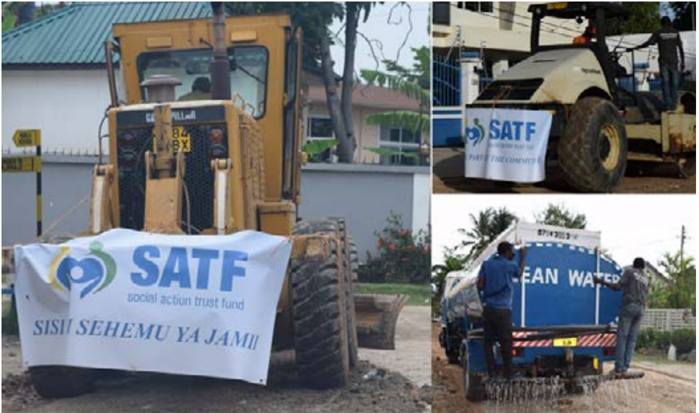
“Sisi ni sehemu ya jamii”-we walked our talk! 5-streets (Manyara Street, Maji maji Street, Daima Street, Ruvu Street and Sangara Streets), were repaired as part of 20th Anniversary celebrations.
